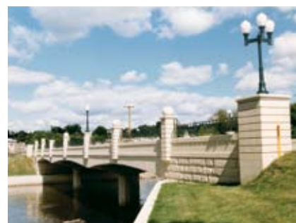
TH 57 over the South Branch of the Middle Fork of the Zumbro River, Mantorville. (Three-span, post-tensioned slab)
