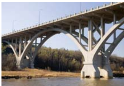
Mendota Bridge, TH 55 over the Minnesota River. (Nineteen-span cast-in-place concrete spandrel arch bridge)
