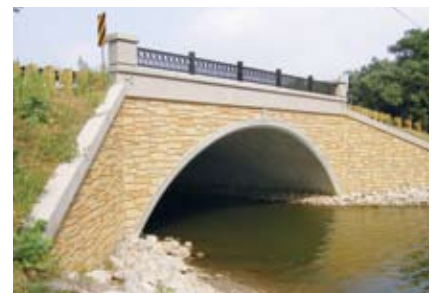
Arcade Street over Channel at Spoon Lake, St. Paul. (Precast concrete arch)
