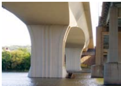
Wakota Bridge, I-494 over the Mississippi River. (Five-span cast-in-place segmental concrete bridge)
