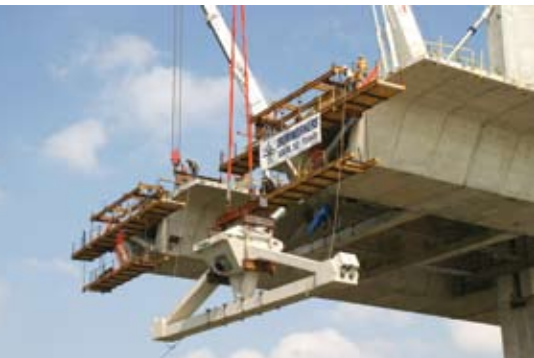
Erection of a precast concrete delta frame that transfers the loads from the segments to the cables.
