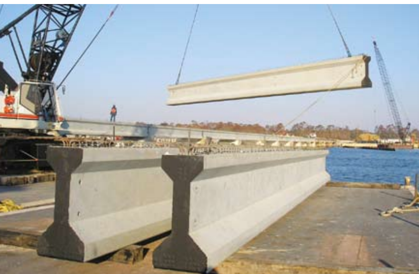
The AASHTO Type IV precast, prestressed concrete beams were erected at an average of 15 beams per day.
