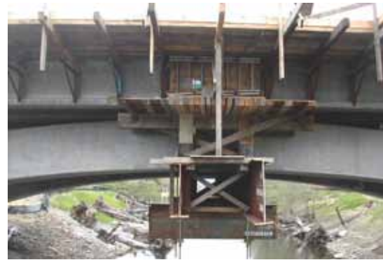
Support for the precast concrete girders was provided at the arched superstructure's apex with a cast-in-place concrete crossbeam.
