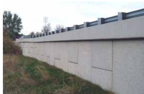
A total of about 18,000 ft 2 of walls were used on both approach fills.
