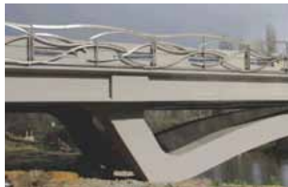
The shape of the substructure arch is flat enough that it functions partially as an arch and partially as a beam. It was cast in one continuous pour to ensure a smooth surface.
