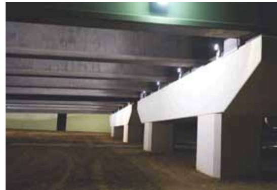
Light is reflected off the underside of the Biloxi Bay Bridge deck, providing sufficient illumination for the pathway and circulation area and making pathway-specific lighting unnecessary.
