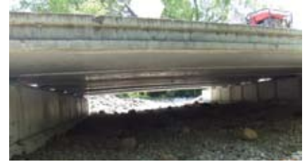
A culvert-replacement project over Lackamas Creek reused bridge slabs obtained from the City of Olympia, where they had been used for a temporary bridge.
