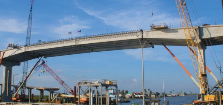
The last 178-ft drop-in girder being erected. Each drop-in girder was cast in two segments, which were transported to the site and then spliced before erection.
