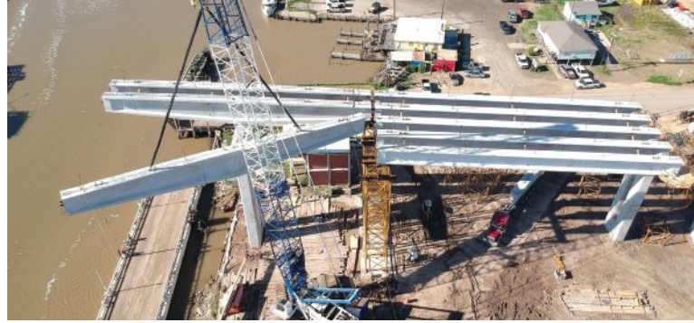
The 120-ft-long, variable-depth pier girder is erected onto the pier and stabilized with a tie-down plate connection to the end girder at the falsework tower.
