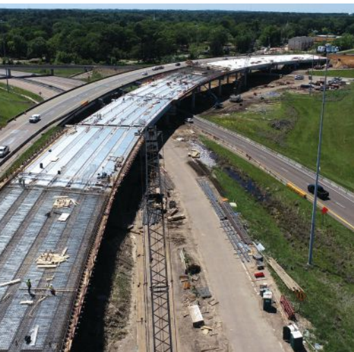
Aerial view of the bridge under construction looking west toward bent 1. Prestressed concrete beams have been erected and stay-in-place deck forms and deck reinforcement have been placed. Photo: Mississippi Department of Transportation.
