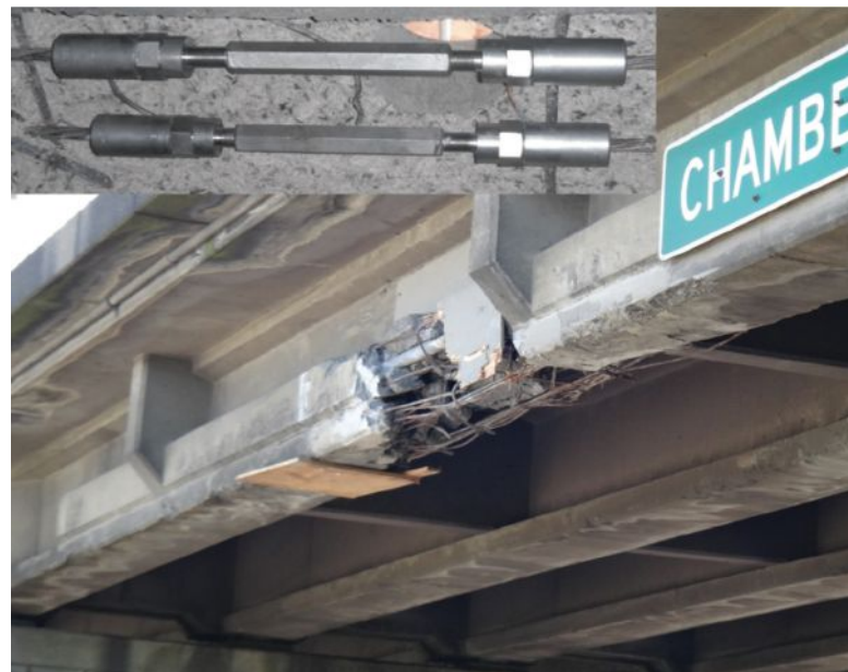
Figure 2: Before the 2016 collision, the same bridge had been damaged at the same location. The severed prestressing strands were repaired using strand splices (shown in inset photo and visible in the first girder in Fig. 1).
