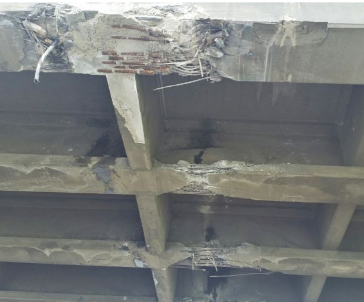
Figure 1: In July 2016, a collision by an overheight vehicle damaged the prestressed concrete girder bridge over southbound Interstate 5 at Chamber Way in Chehalis, Wash. All Photos: Washington State Department of Transportation.
