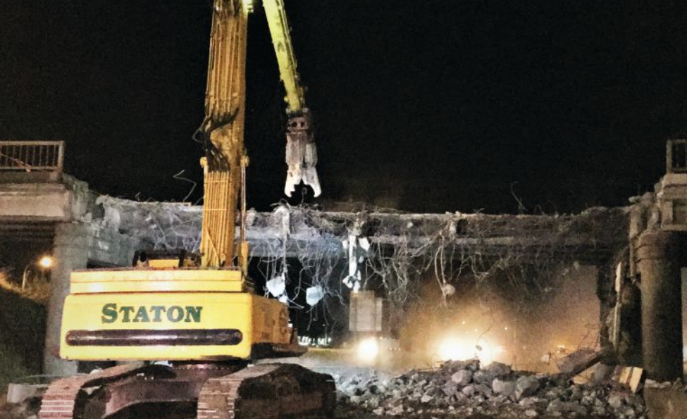
Figure 3: Because significant structural damage was incurred during the 2016 collision, the Washington State Department of Transportation demolished the damaged span in its entirety and installed a temporary bridge until the replacement span could be constructed.
