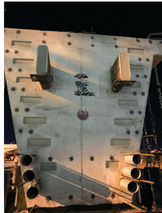
Drop-in girder segment (girder segment 3) arriving on site. The corbels projecting from the end diaphragm with bearing plates on bottom are higher in the section so they can rest on the corbels in the pier segments. Shear keys and embedded couplers for installing mild reinforcement for the splice are visible on the end of the girder. Photo: Modjeski and Masters Inc.
