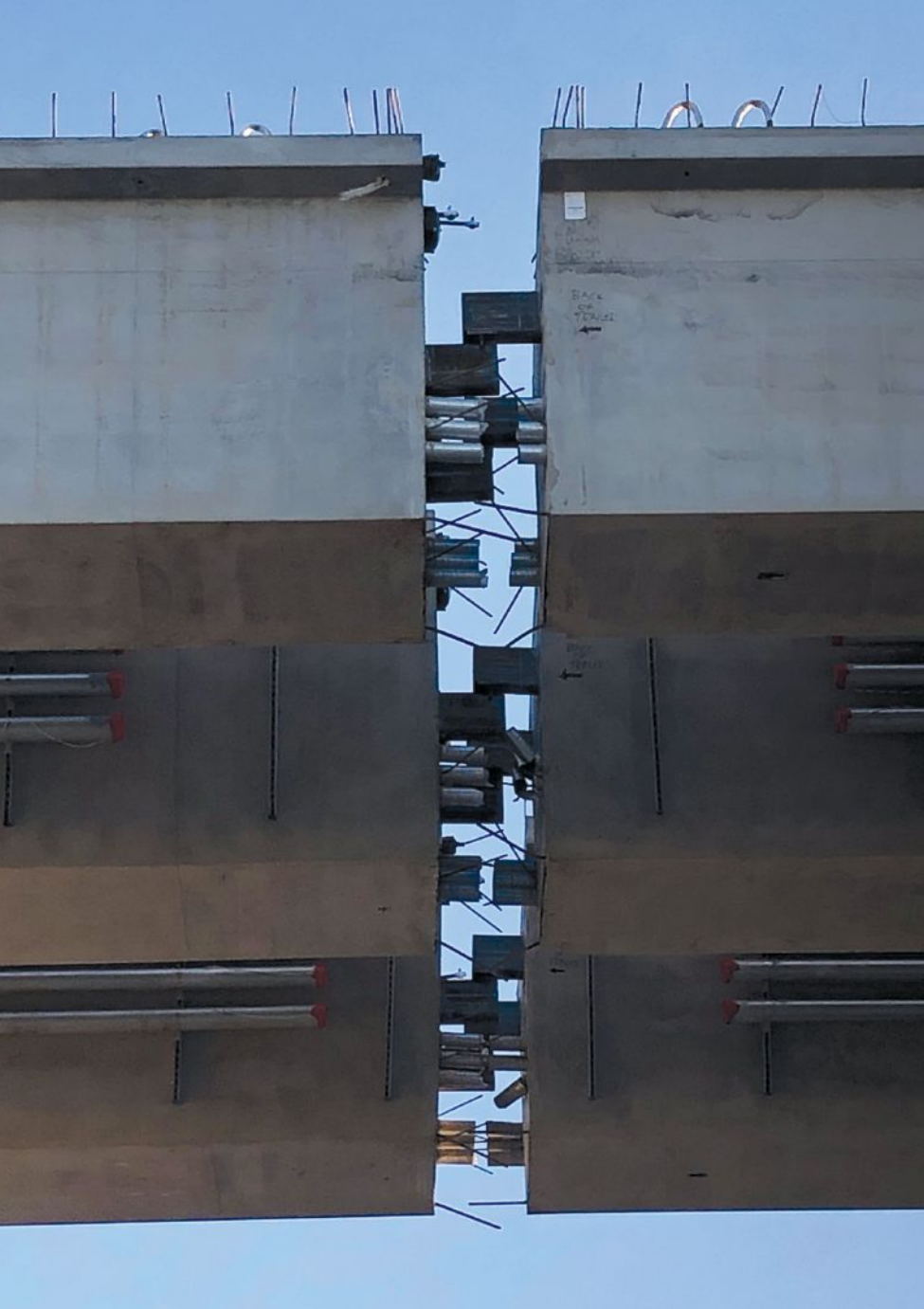
Embedded corbels projecting from drop-in girder segments, here shown at right, resting on corbels projecting from cantilevered ends of girder segments on left. Photo: Hensel Phelps.
