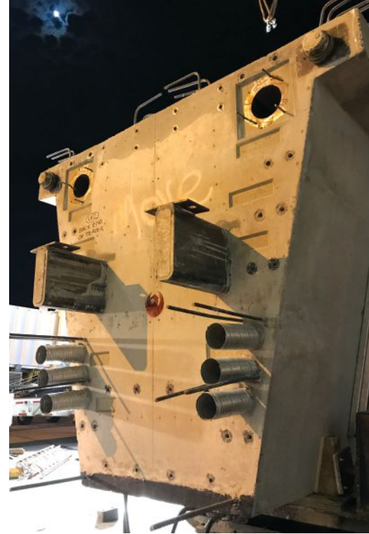
Pier girder segment after arriving on site. The corbels projecting from the end diaphragm with bearing plates on top are lower in the section to support the corbels for the drop-in segment. Post-tensioning anchors are located near the top of the diaphragm for first-stage post-tensioning tendons. Smaller, plant-installed post-tensioning tendons are located at the top outer edges of the section. Photo: Modjeski and Masters Inc.
