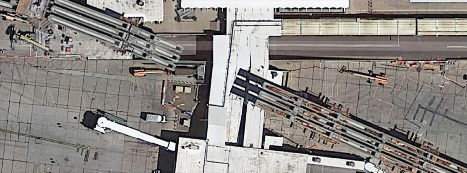
Overhead view of the construction site before drop-in segments were erected over Terminal 2. Splices and pier diaphragms are visible. Photo: Google.
