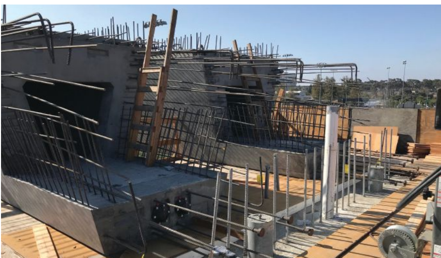
Girder segment with blockout for closure pour and post-tensioning anchorage hardware. This photo also shows both pins in the pier cap. Photo: WSP.
