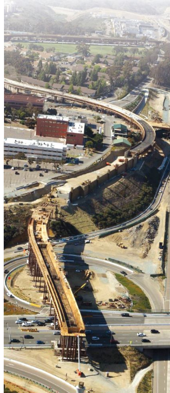
Mid-Coast Transit Corridor alignment near the San Diego VA Medical Center. Photo: Mid-Coast Transit Constructors.
