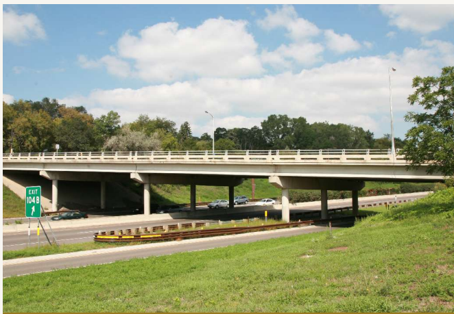
Migrating corrosion inhibitors were tested in an overlay repair on the Randolph Avenue Bridge in St. Paul, Minn. Photo: Cortec Corporation.
