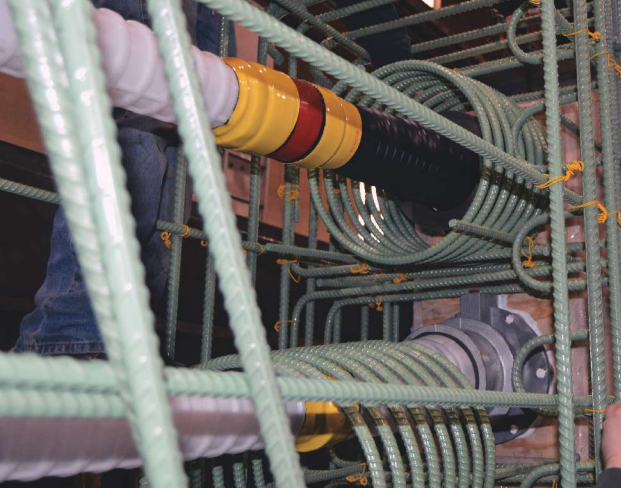
Post-tensioning anchorages in precast concrete beams during spiral reinforcement installation, with an electrically isolated tendon trumpet (top) and a traditional trumpet (bottom).
