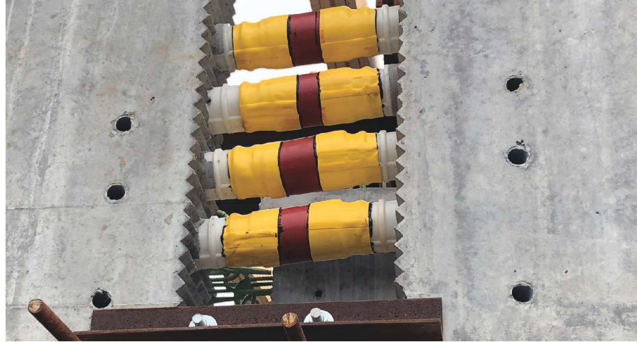
Post-tensioning splice prior to placement of the closure joint. No difference can be seen between the electrically isolated tendon at the top and the three conventional tendons below.
