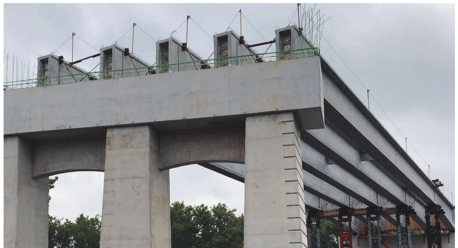
The main unit of the Coplay-Northampton Bridge consists of a 540-ft-long, three-span section over the Lehigh River. The superstructure consists of five prestressed concrete PA bulb tees, which were spliced and post-tensioned. All Photos: Dr. Clay Naito.
