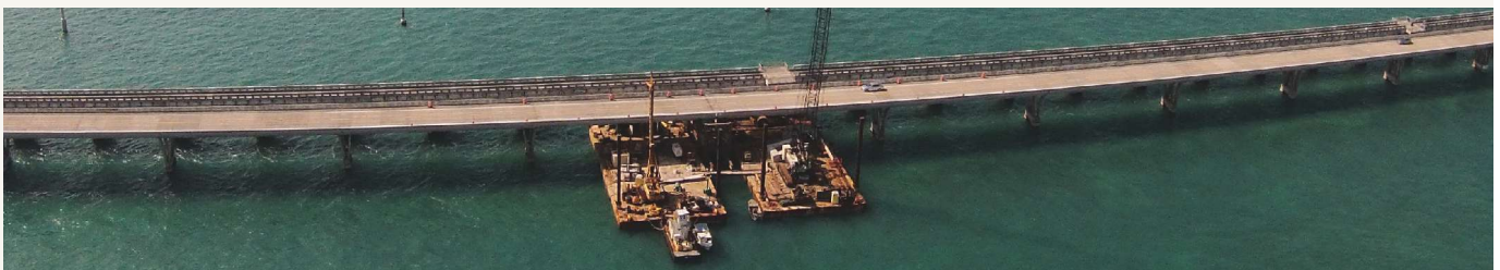
Aerial view of the barges in position for V-pier installation. All Photos: James Charles.
