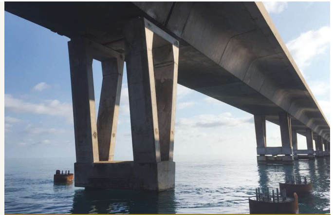
New V-pier installed. The 48-in.-diameter drilled shafts used for the temporary support system installation can be seen. These were later removed to 1 ft above the mudline.
