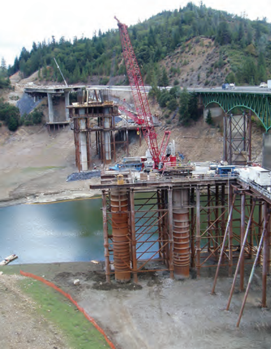
Construction casings and access trestles were built when the lake was full but are exposed when the lake is low.
