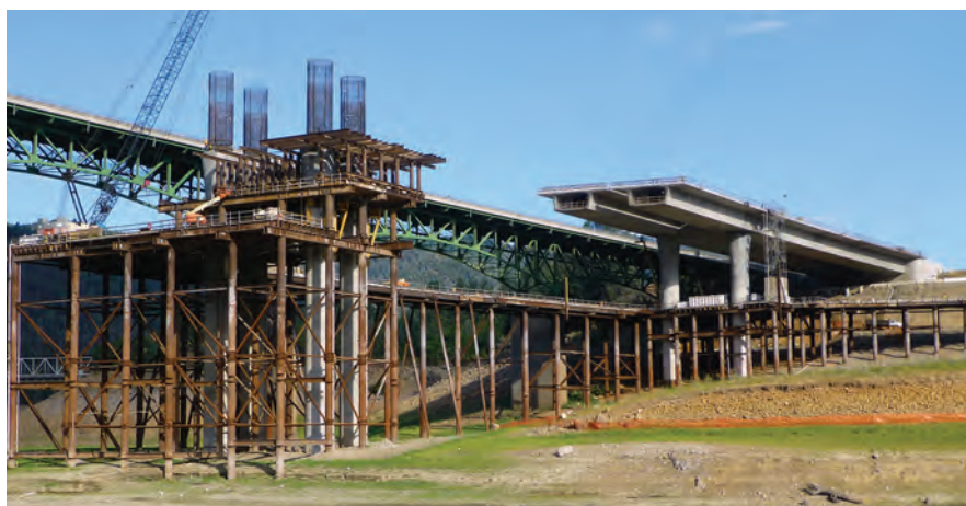
Drought left the access trestle high and dry.
