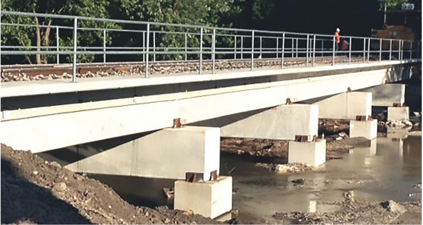
Precast concrete subcaps, caps, and double-cell box beams at Barstow, Ill. Replacement took place during a 16-hour track closure. Photo: BNSF Railway.
