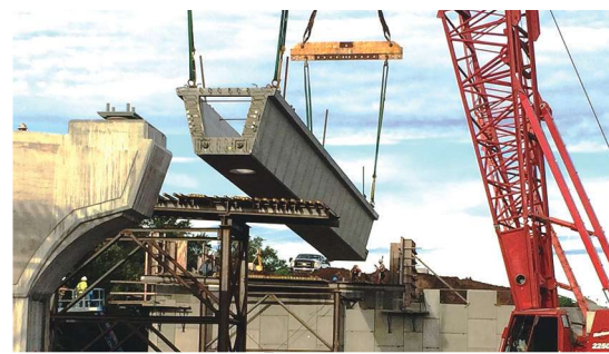
First Ramp H girder being lifted into place, supported by abutment and shoring tower. Photo: A2 Group.
