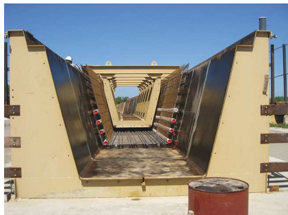
View of curved forms with reinforcing steel and core form in place. Photo: Parsons.
