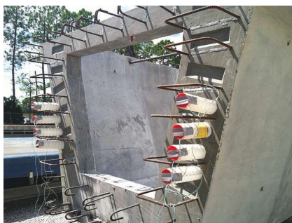
View of typical girder end details, including thickened webs, top strut, shear keys and reinforcing steel to be tied with closure placement reinforcement. Photo: Parsons.
