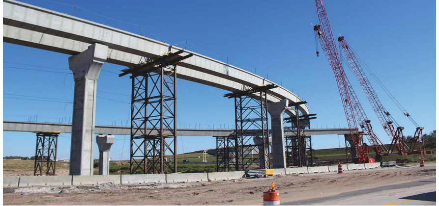
View of erected Ramp I girders spanning above Ramp H. Photo: Parsons.
