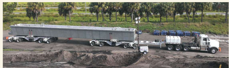
Girder at site ready to be lifted into place. Photo: Dura-Stress Inc.
