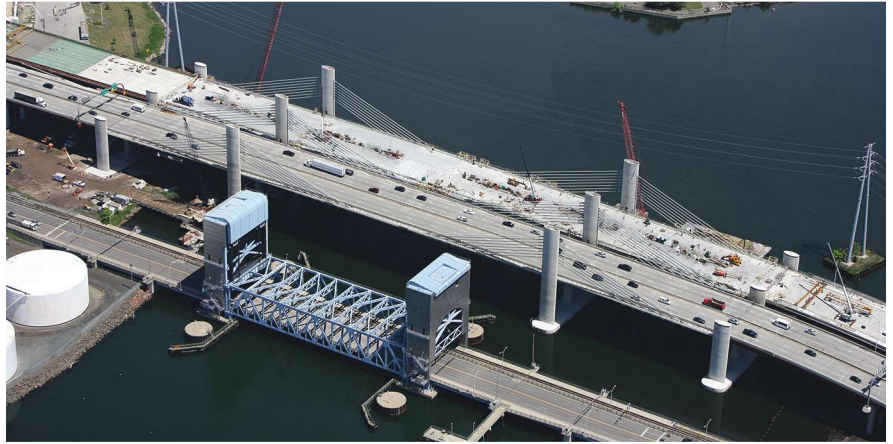
Aerial photo of the cable-stayed main span. Photo: Walsh-PCL JV II and Shoreline Aerial Photography.
