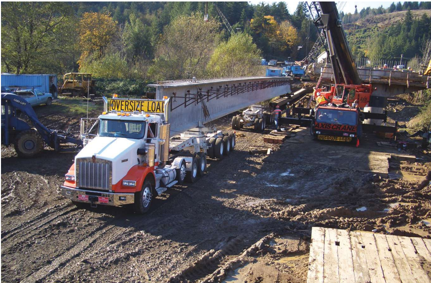
Single-span girder launching system where truck pushes girder across the launching girder. Photo: Knife River Corporation.
