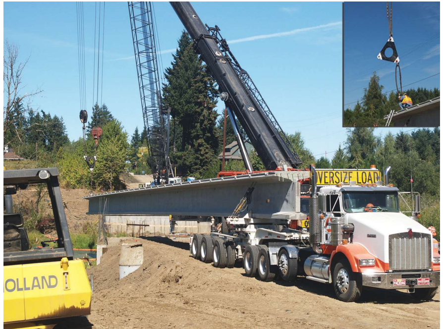
Passing a girder between two cranes using a load triangle (inset). Photos: Knife River Corporation.
