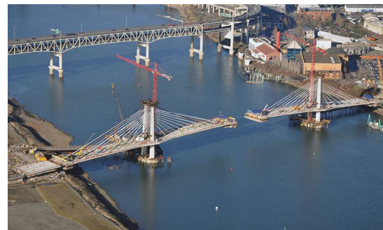
Balanced cantilever construction with work bridges to the main pylons to deliver material to the four construction fronts at the tips of the cantilevers. Photo: Sahnov’s Air Photos, Banks, Ore.
