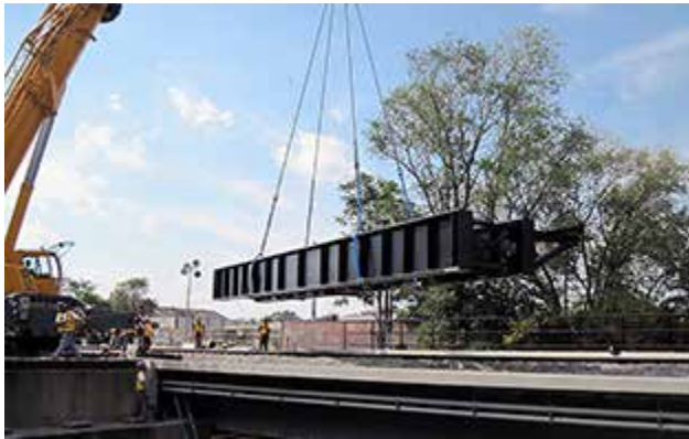
Elevation of prefabricated steel plate girder, picked up by crane over the bridge at mile
