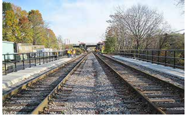
North approach view of the two main tracks looking north on bridge 2 over the Neponset River bridge.
