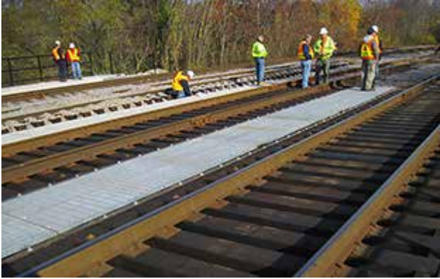
Top surface view of two main tracks and two spur tracks on bridge 1 over the Neponset River. All photos: The Louis Berger Group Inc.
