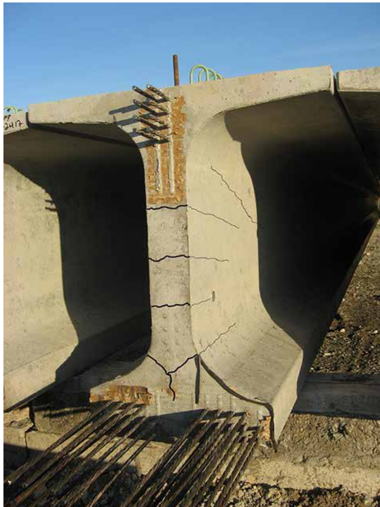
Girder end cracking that developed during the prestressing process. Photo: Wisconsin Department of Transportation.
