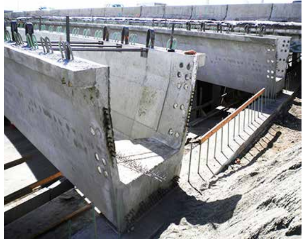
The superstructure consists of U72 precast concrete girders. All Photos: Summit Engineering Group, Inc.
