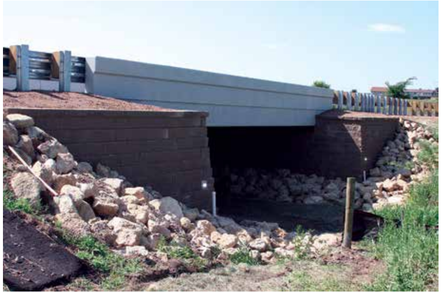
Accelerated bridge construction demonstrated with a geosynthetic reinforced soil-integrated bridge systems structure. All photos: Wisconsin Department of Transportation.
