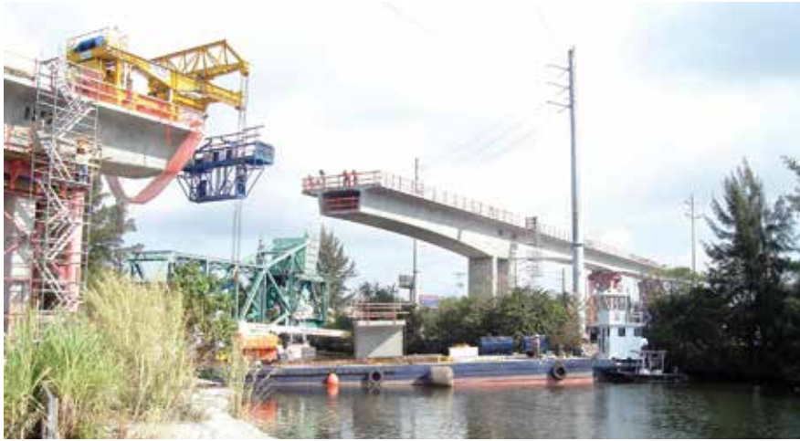
The Miami Intermodal Center—Earlington Heights Connector features three types of concrete spans, including precast, post-tensioned segmental concrete box girders. Thirteen single-cell, constant- and variable-depth box girder units were erected using the balanced cantilever method. Photo: Rizzani de Eccher USA.
