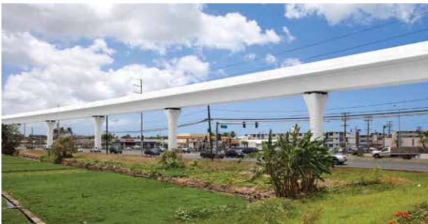
The Honolulu High-Capacity Transit Corridor Project for the Honolulu Authority for Rapid Transportation, currently under construction, features single-cell trapezoidal box girders to carry a dual track. This rendering shows the Kamehameha Highway section of the project. Photo: FIGG.
