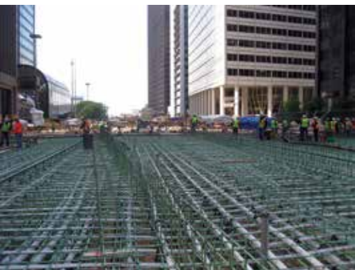
The rebuilt two-level Wacker Drive viaduct in Chicago replaced the existing 1400-ft-long structure but retained many of the existing caissons. To help attain a 100-year service life, the deck slab was post-tensioned in both directions and included epoxy-coated reinforcement.
