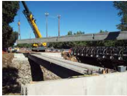
Precast, prestressed concrete box beams that were 106 ft long, weighing 106,000 lb, were set with two cranes from the abutments. Traffic was stopped seven to 15 minutes to make picks from the temporary bridge.
