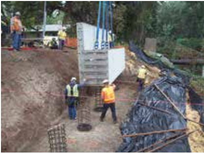
Each precast concrete abutment was fabricated in two pieces, with each piece weighing 72,000 lb.
