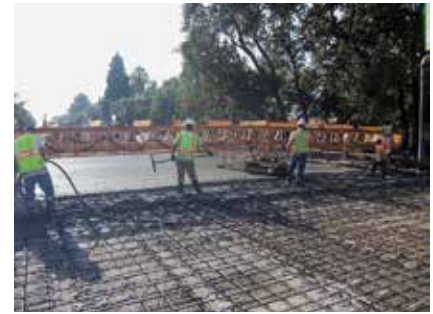
Cast-in-place, high-performance concrete deck being placed using a concrete mix containing a shrinkage-reducing admixture and macro fibers.
