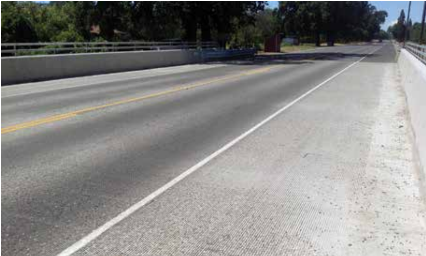
Craig Creek Bridge deck shows no cracking nearly two years after construction completion. Deck concrete contains a shrinkage-reducing admixture and fibers, and was subjected to a shortened curing period.
