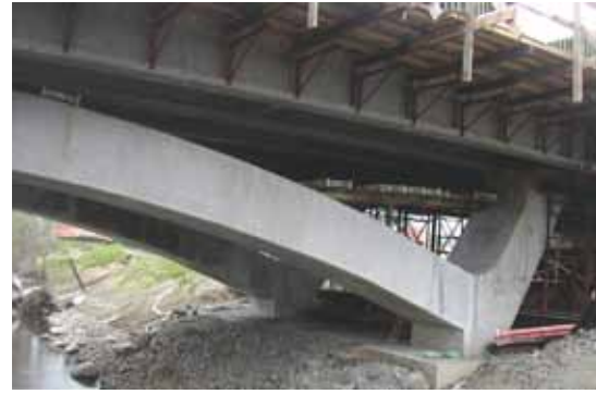
To provide a robust foundation for the columns on both sides, 120-ft-long cast-in-pipe concrete piles were used to carry both gravity loads and thrust from the arch. At each column pier, a crossbeam was constructed on falsework to support the precast concrete girders and deck.
