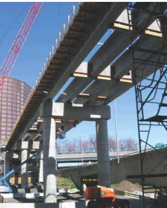
Four lines of bulb tees were used in the superstructure with cast-in-place concrete diaphragms. Photo: Purcell Associates.
