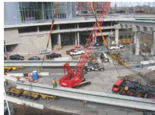
The heaviest pick was approximately 50 tons. Interstate highway on-ramps were temporarily closed to allow for beam delivery and erection. Photo: Purcell Associates.
