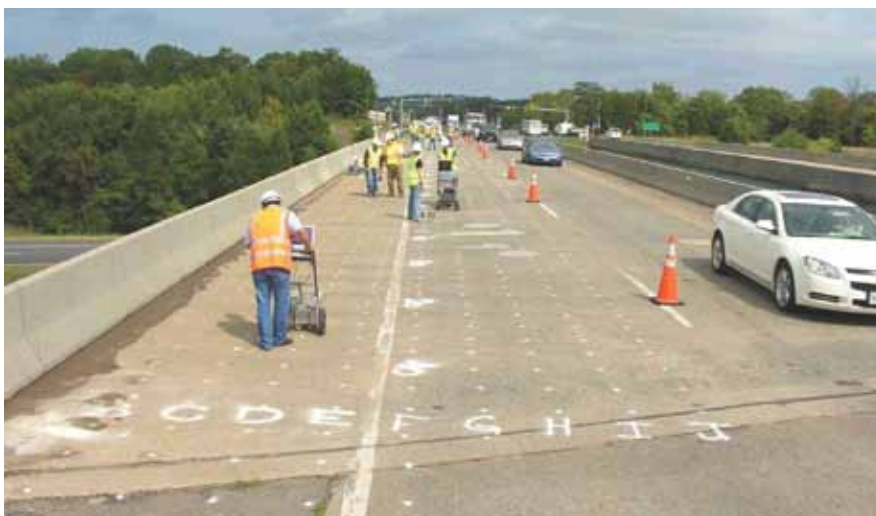
Deck delamination repair before application of an overlay. All photos: Virginia Department of Transportation.
