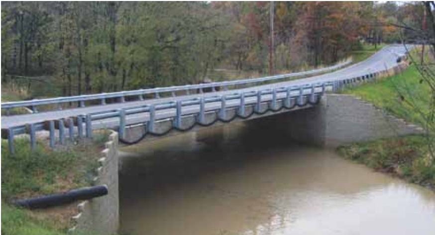
The Bowman Road Bridge was the first GRS bridge constructed by Defiance County in 2005. It uses an 80-ft-long beam. The bridge is 34 ft wide with a 24-degree skew and 7.6-degree superelevation. The abutments are 43.6 ft long and 15.25 ft tall.
