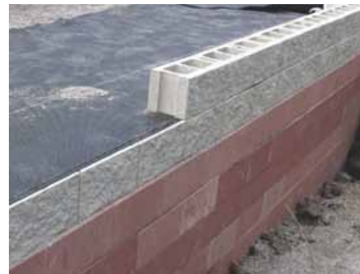
A close view of the 8-in. concrete masonry units forming the face of the abutment and the geotextile between layers.
