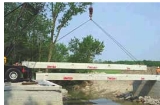
Adjacent precast, prestressed concrete box beams are placed directly on the geotextile covering the compacted granular backfill.
