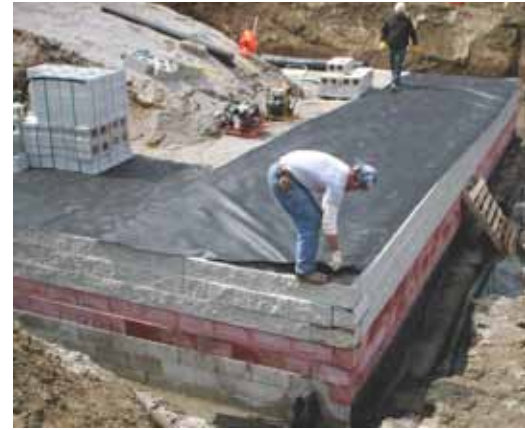
A geosynthetic reinforced soil (GRS) abutment is constructed in 8-in.-high lifts with a layer of geotextile between each lift.
