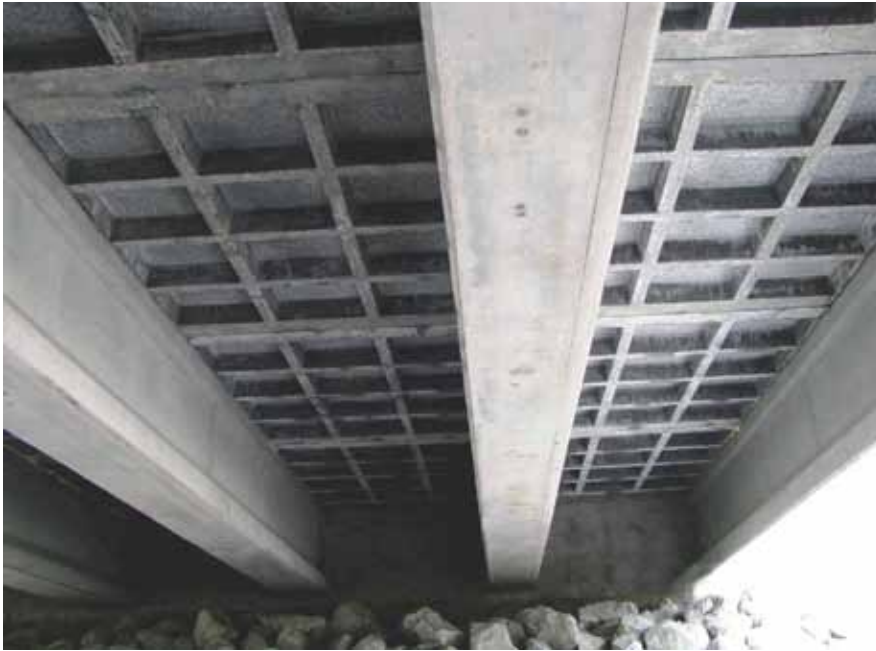
The underside of the completed Little Cedar Creek Bridge showing ultra-high-performance concrete (UHPC) waffle panels on conventional precast, prestressed concrete I-beams. All photos: Wapello County.
