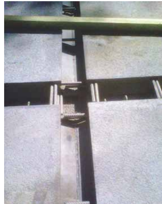
Short extended reinforcing bars are shown in the longitudinal and transverse joints prior to placing the UHPC field-cast closures.
