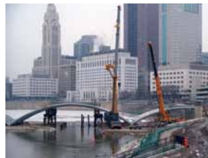
Snow flurries did not stop construction of the top segment of the rib arch on the Rich Street Bridge. Photo: Ohio Department of Transportation District 6.
