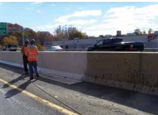
Application of elastomeric paint to a median barrier. Photo: Federal Highway Administration.
