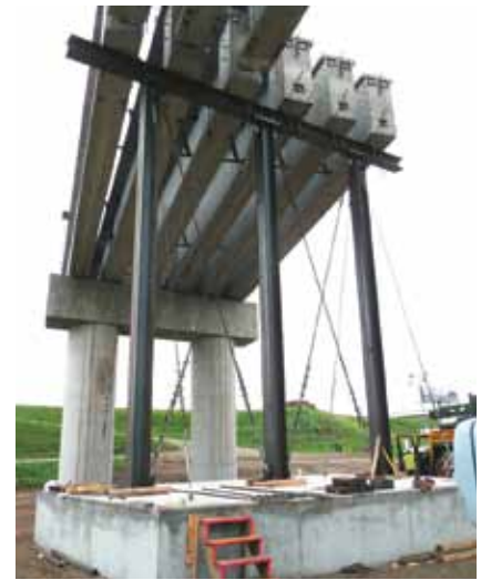
Girder segments D supported on temporary bent with E-girder segments partially constructed supported by overhead strongbacks.
