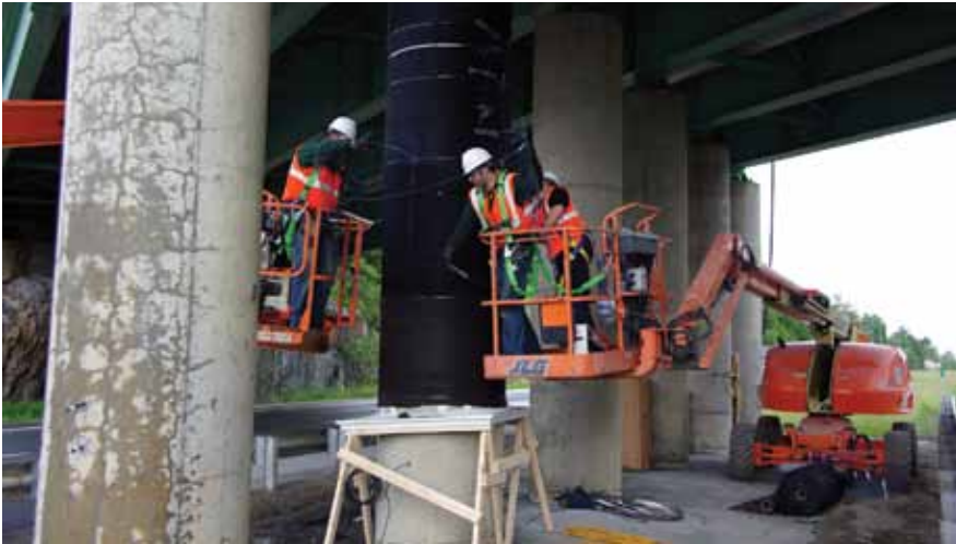
Application of Carbon Fiber Reinforcement Polymer (CFRP) wrap to a bridge column. Photo: Federal Highway Administration.
