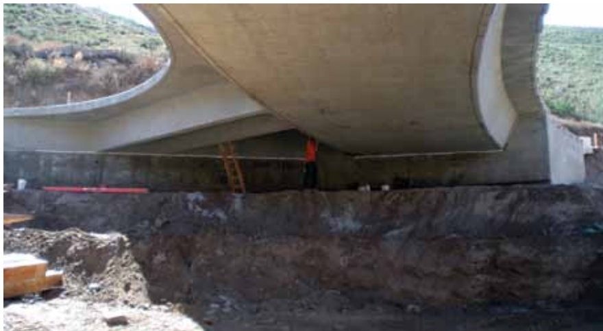
From below, shown is the framing between Sutherland Dam Road and Black Canyon Road. Photo: County of San Diego.
