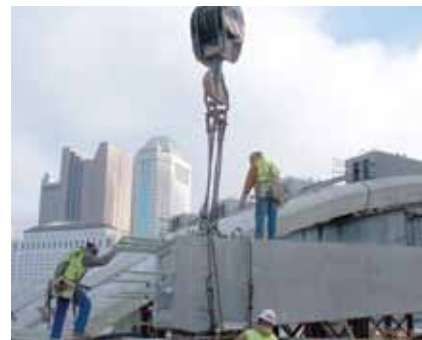
Delivery of the precast, prestressed concrete girders. Photo: Ohio Department of Transportation District 6.
