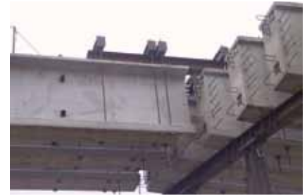
Girder segments A, C and E are supported using overhead strongbacks prior to the cast-in-place concrete closures being cast.
