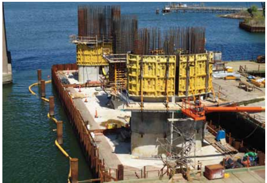
Tower leg jump-form systems were sprayed with insulating foam to control thermal gradients during mass concrete curing. Photo: Lochner/FIGG.
