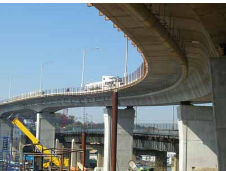
Precast concrete footings, piers, and superstructure segments were used to accelerate construction on the Route 36 Highlands Bridge. Photo: J. H. Reid General Contractor, Unistress Corporation, or DYWIDAG-Systems International USA Inc.
