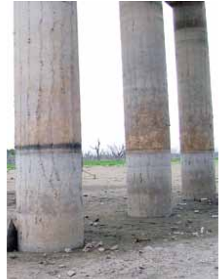
Signs of ASR-induced damage. Photo: Courtesy of Texas Department of Transportation. Copyright © 2002. All rights reserved.
