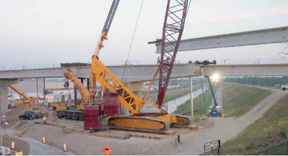
The crane was positioned on a temporary crane pad to protect critical utilities below.
