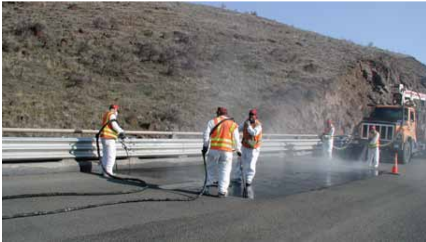
Deck sealing was completed by Oregon Department of Transportation bridge maintenance crew. Photo: Oregon Department of Transportation.
