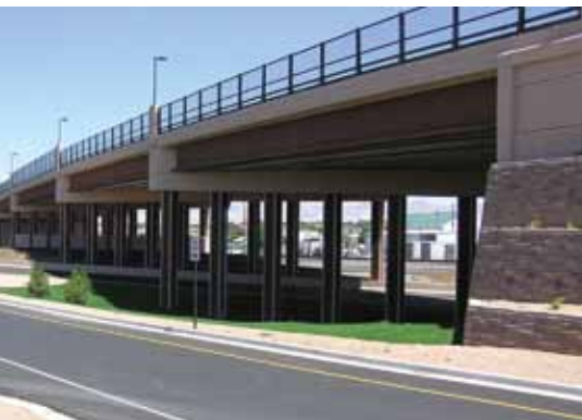
The Riverside Parkway project also included a prestressed concrete bridge over the Union Pacific Railroad at 25 Road.
