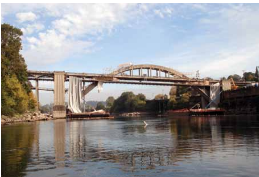
A complex rehabilitation project of the Oregon City Arch Bridge used an innovative, custom shotcrete mix specifically designed to adhere to the existing steel.
