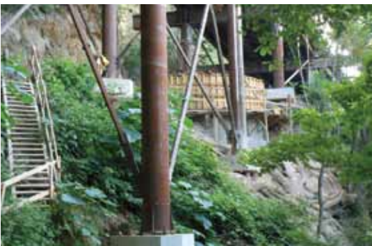
View below the temporary work trestle, as pier 1 footing is formed on top of the sub-footing concrete.
