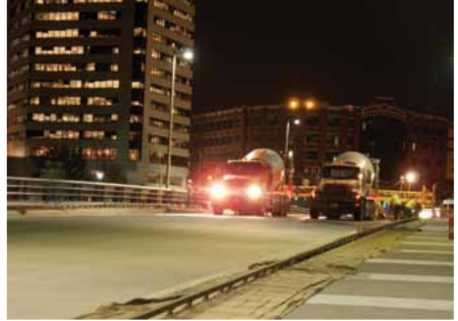
Placement of the 1½-in.-thick silica fume overlay on the bridge deck. Photo: Ohio Department of Transportation District 6.
