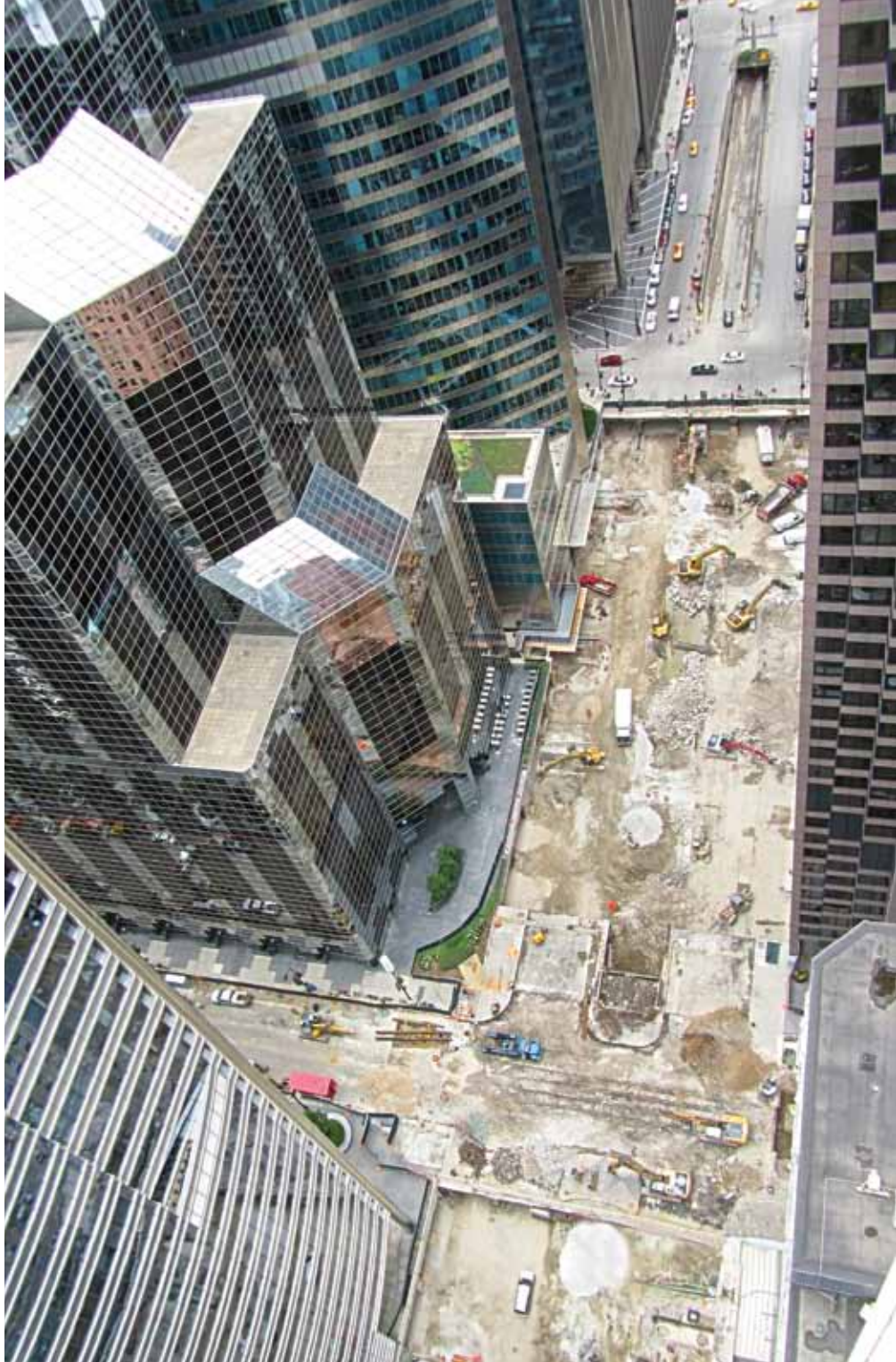
View from adjacent skyscraper looking down on the existing Madison Street intersection prior to completing deck demolition. Photo: McHugh Construction.
