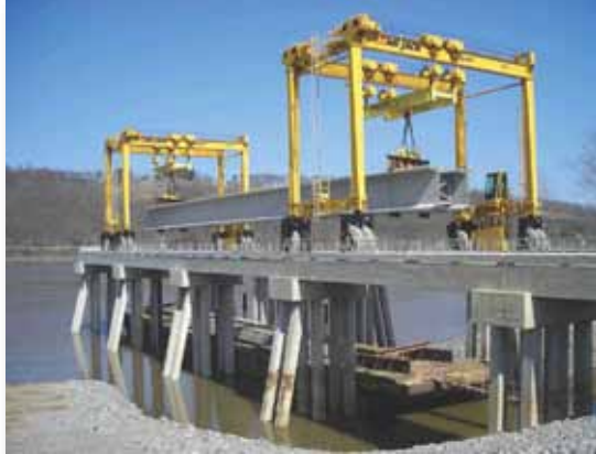
Above: The precaster's loading pier allowed the heavy precast girders to be placed on specially designed barges, which delivered the components to the site. The 185-ft-long main-span, drop-in girders were always handled as braced pairs to address stability concerns. Photo: Prestress Services Industries LLC.
