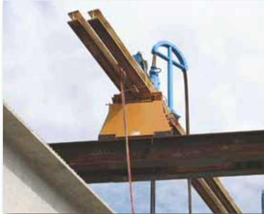
A strand jack was used to lift haunched pier segments from the barge to the pier seats. The jacks were later relocated and used to lift the drop-in girders for the main span. Photo: Haydon Bridge Co.
