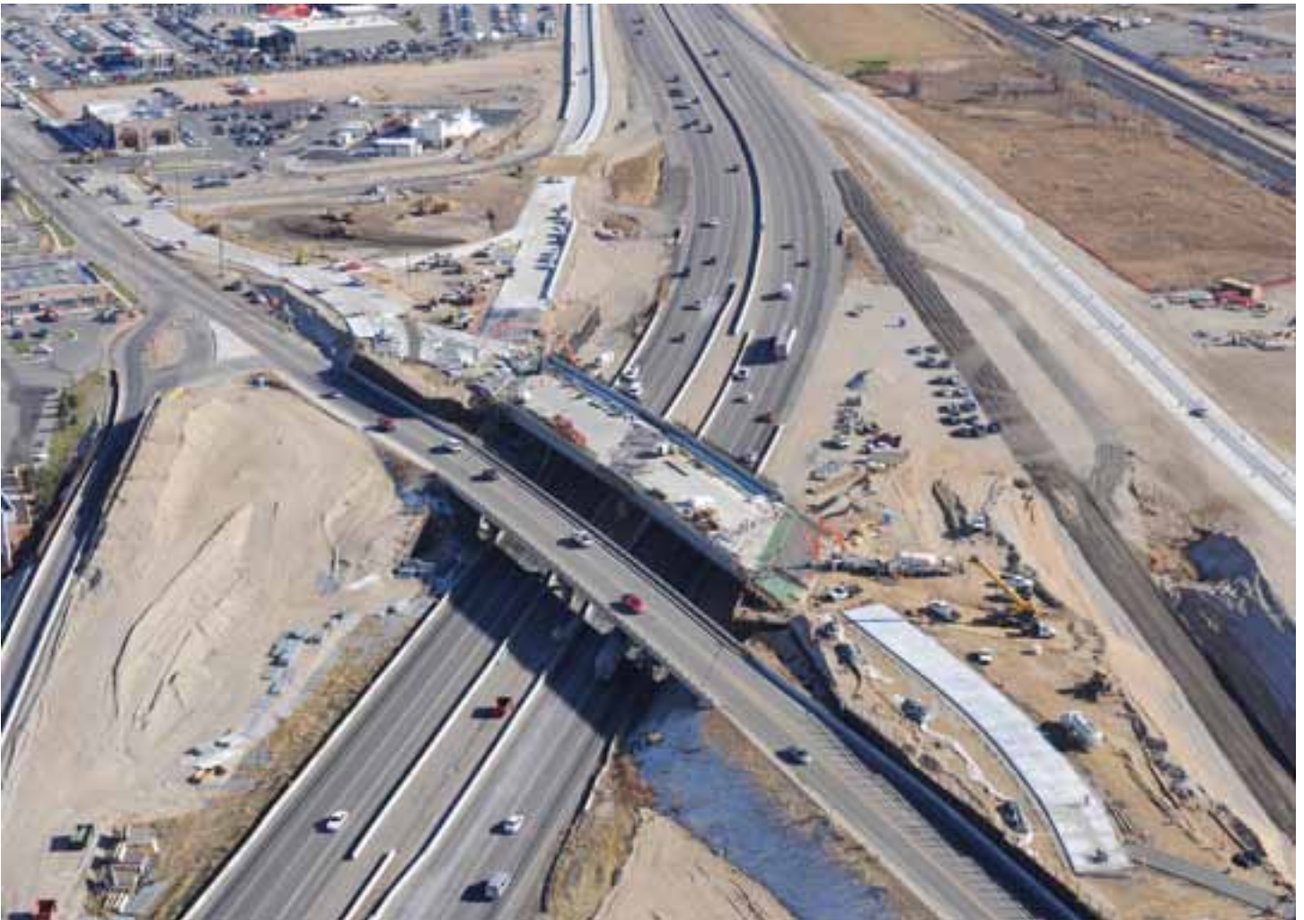
Work being completed on the Phase 1, westbound bridge. Traffic was maintained on the existing structure prior to being moved to the spans placed during Phase 1.
