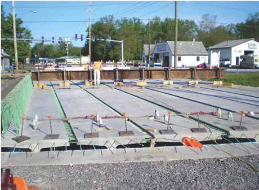
Route 31 over Canandaigua Outlet shown during construction, is a precast, prestressed concrete deck bulb tee ready for the field-cast UHPC joints to be filled.
