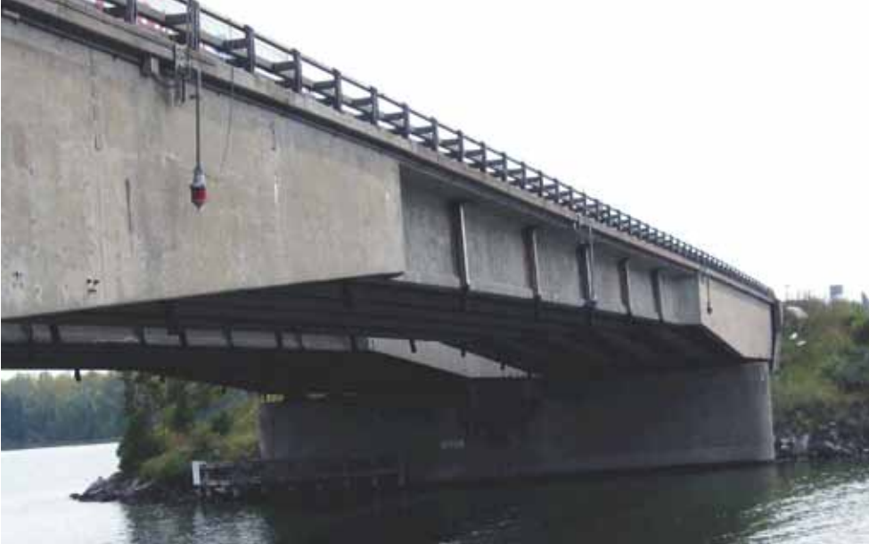
I-81 over Oneida Lake is a precast, post-tensioned concrete, spliced girder bridge. At 320 ft, it was the longest concrete spliced girder span in the world from 1960 until 2010.
