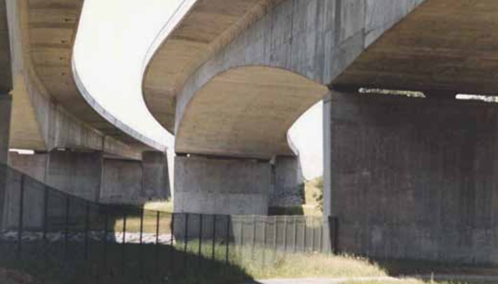
The twin, 2300-ft-long, I-390 bridges over the Genesee River, built in the 1970s, were some of the first cast-in-place, post-tensioned segmental concrete bridges in the United States.
