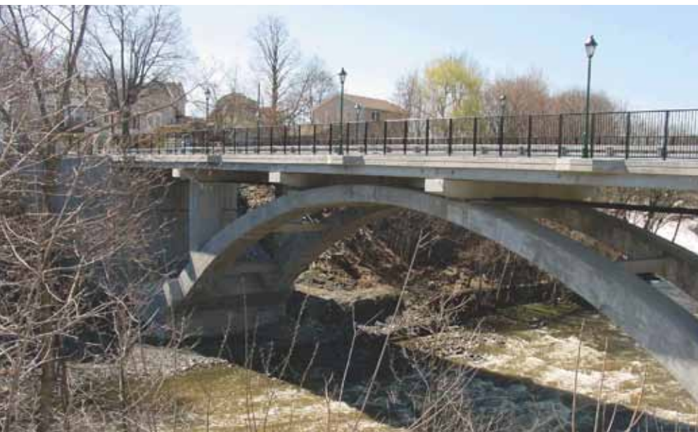
The Route 5S over Wallkill bridge uses cast-in-place, reinforced concrete arches with precast concrete spandrel columns, cap-beams, and a precast, prestressed concrete adjacent box beam superstructure. All precast components were made using self-consolidating HSHPC.
