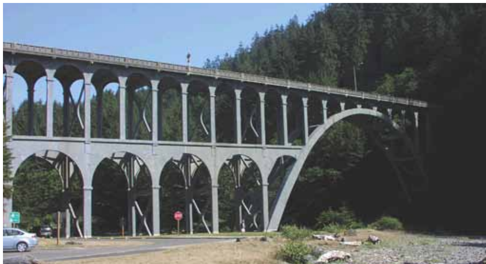
The Cape Creek Bridge on the Oregon Coast Highway is a 619-ft-long, two-tiered reinforced concrete arch inspired by the Roman aquaduct near Nimes, France. The bridge, completed in 1932, is still in use today. Photo: Henry G. Russell.
