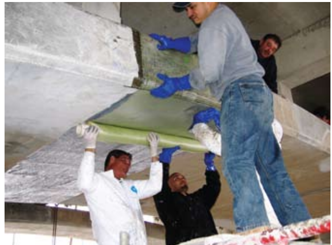
The contractor's low bid on the project allowed city officials to extend the wrapping work to include the center arch and still have the total cost come in below the original engineering estimate.
