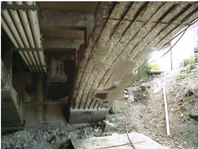
The arches on the bridge, which is listed on the Illinois Historic Bridge List and eligible for the National Register of Historic Places, needed to be repaired so that its historic nature was not disturbed.
